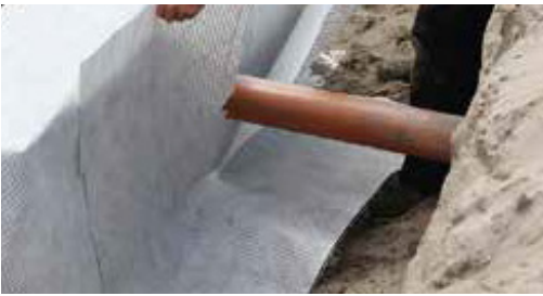
Use another piece of TP combigrd to make cover the cut. This cloth should overlap 1m left and 1m right of the utility.
