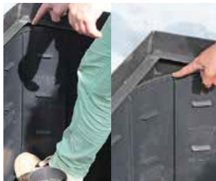
In a open tree pit, the panels should be placed as close as possible to the kerbing. This way you create the maximum space for the tree
