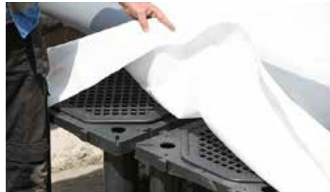
If the height difference is less than 20 cm you can use the standard TP geotextile on top of the system.
